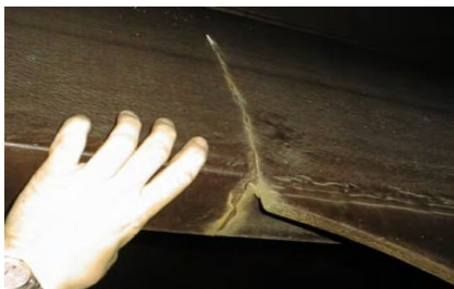
Crack in stiffener
